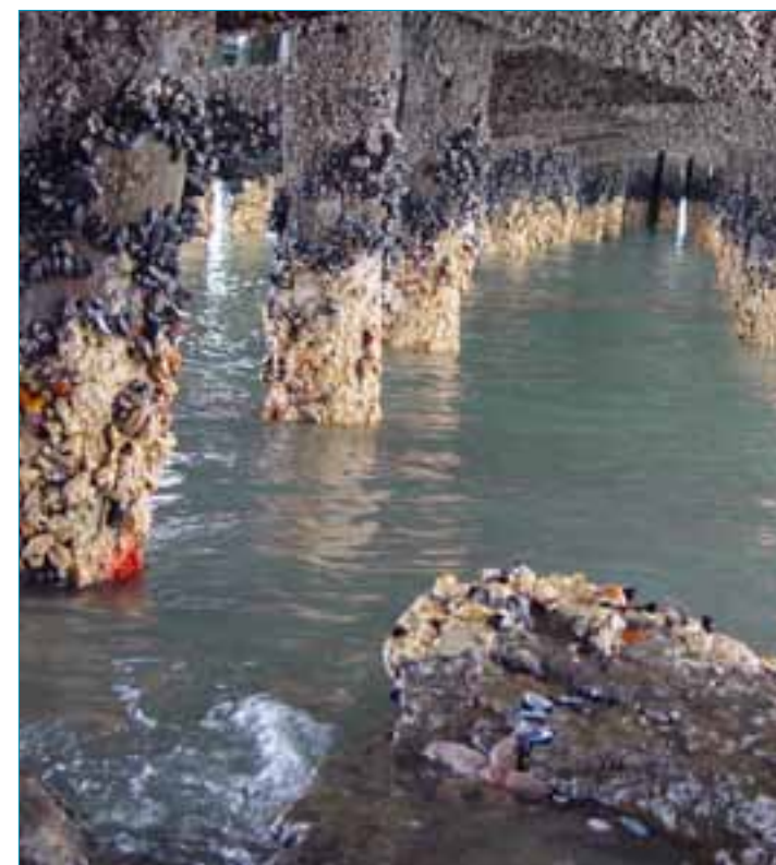
Creosote piling are sources of polycyclic aromatic hydrocarbons.
